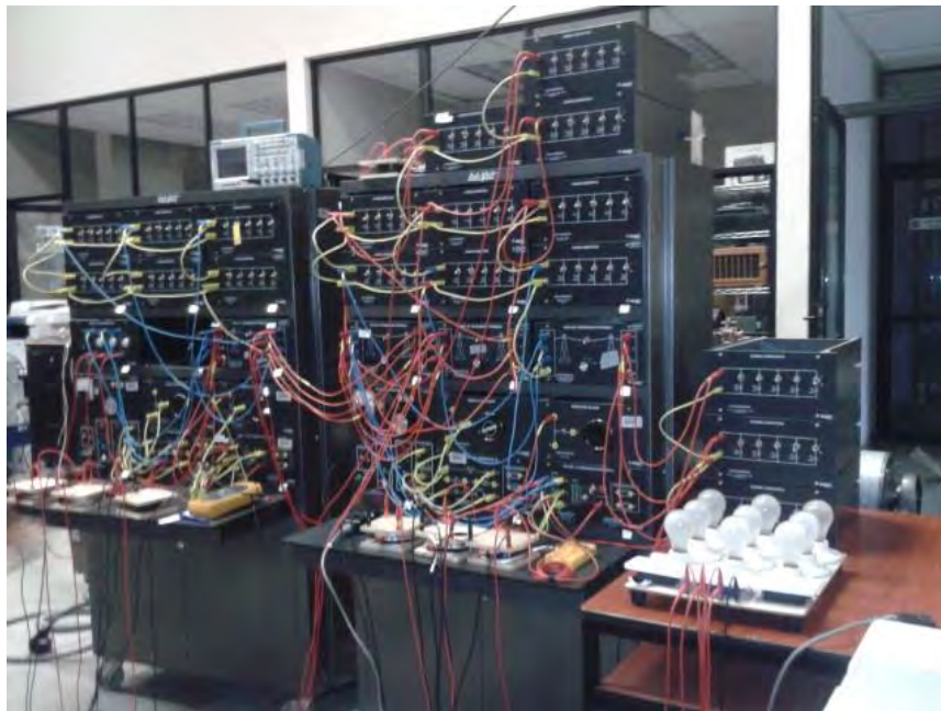
Fig. 2.9 Wired test power system
